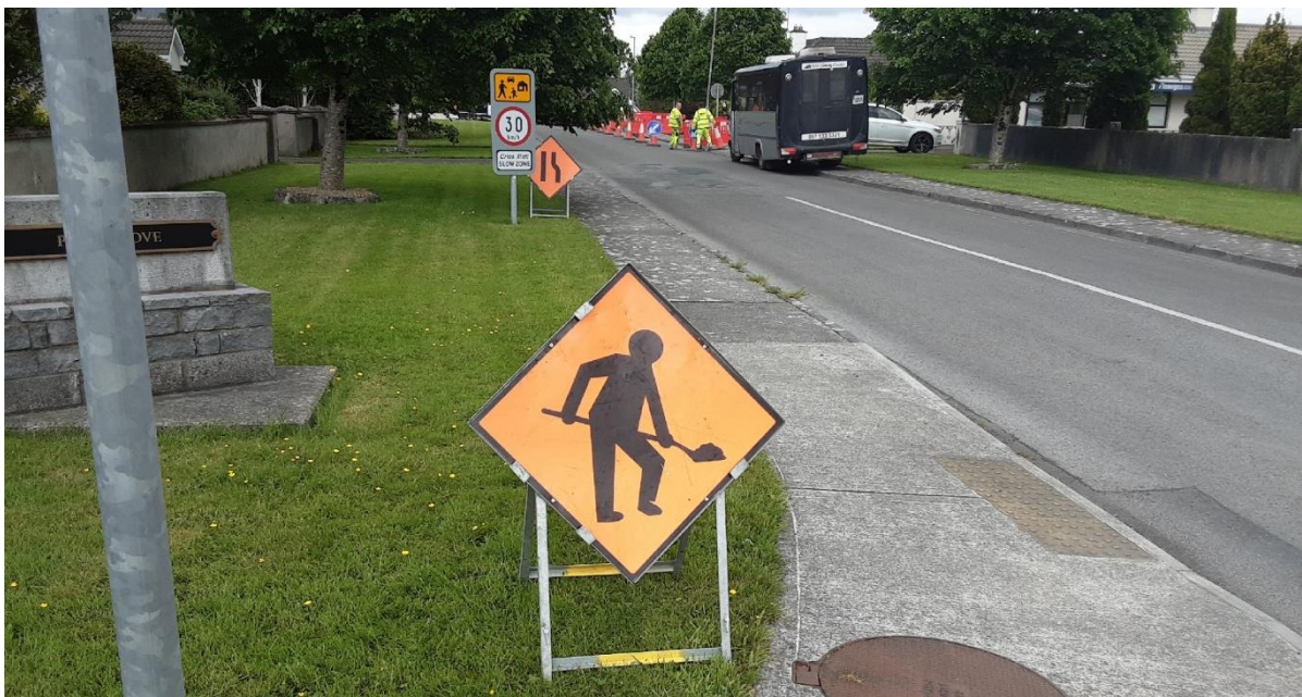
FOOTPATH REPAIRS BEING UNDERATKEN BY BALLINASLOE MD DIRECT LABOUR CREWS AT PINEGROVE MOUNTBELLEW
