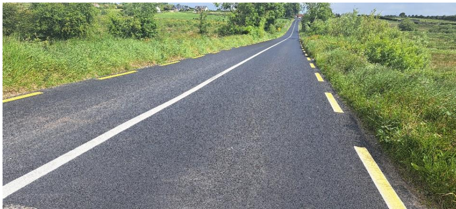
ROADSTONE CONTRACTORS - RI RESTORATION IMPROVEMENT, AT ARDEEVIN R364 - 2024 ROADWORKS PROGRAMME BALLINASLOE MD
