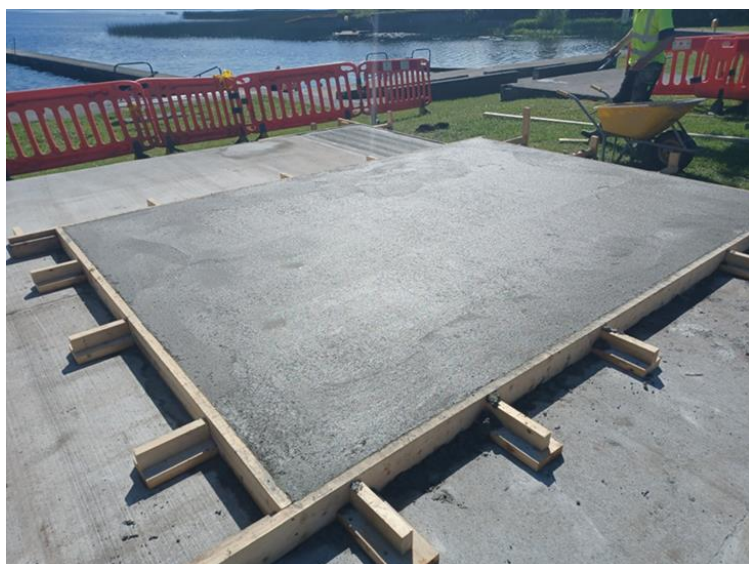
CONSTRUCTION OF CONCRETE BASE FOR NEW LIFEGUARD HUT AT PORTUMNA SWIMMING AREA
